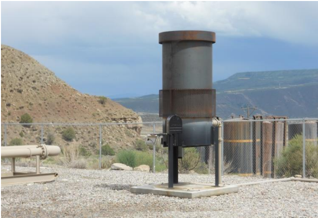
A combustion device and storage tanks EPA photo
