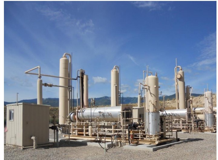
Glycol dehydrators at a well production pad EPA photo
